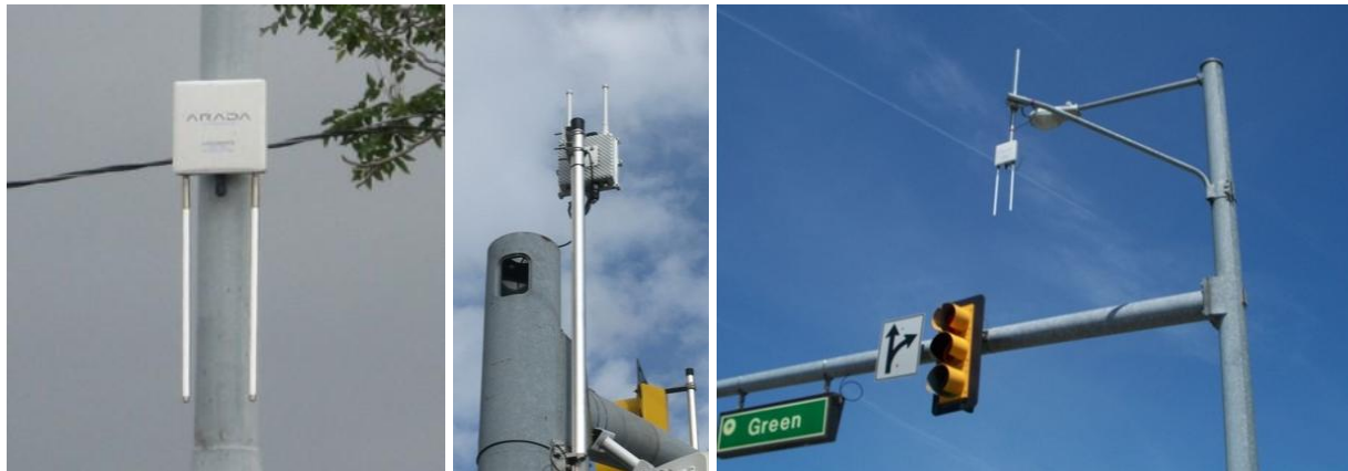
Figure 2: Example Pictures of Roadside Units for Dedicated Short-Range Communications Broadcast
